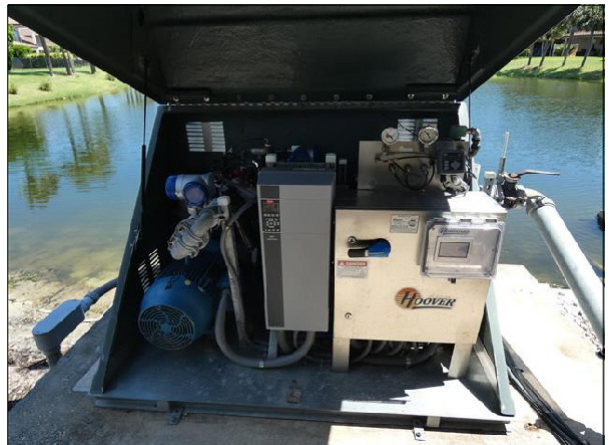
Pump Station 1 Montecito Dr
