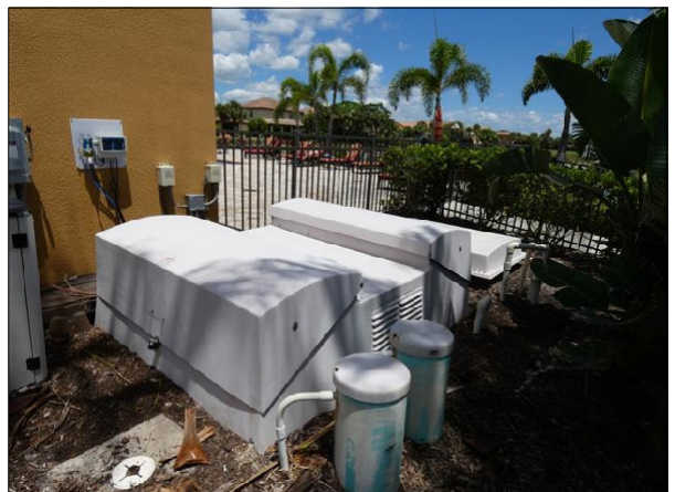
Pool Equipment Housing Boxes
