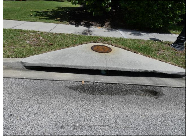
Stormwater Drainage Curb Inlet
