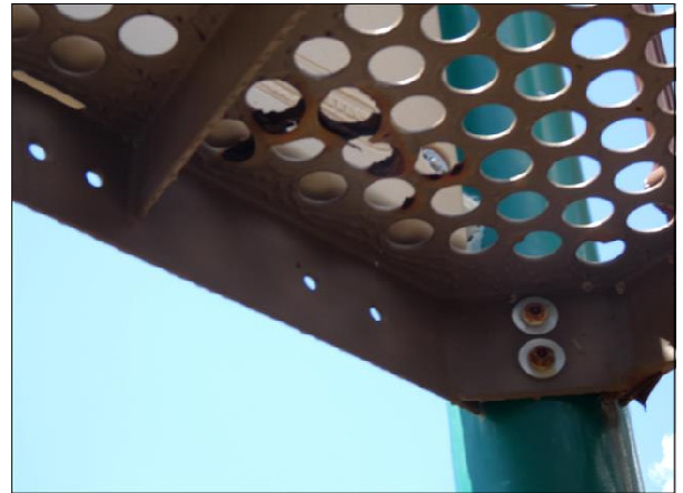
Playground, Note Rust
