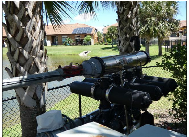
Pump Station 3 Carlsbad Dr
