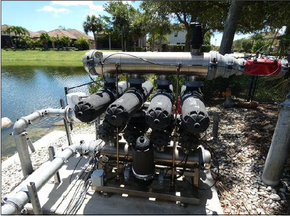
Pump Station 1 Montecito Dr
