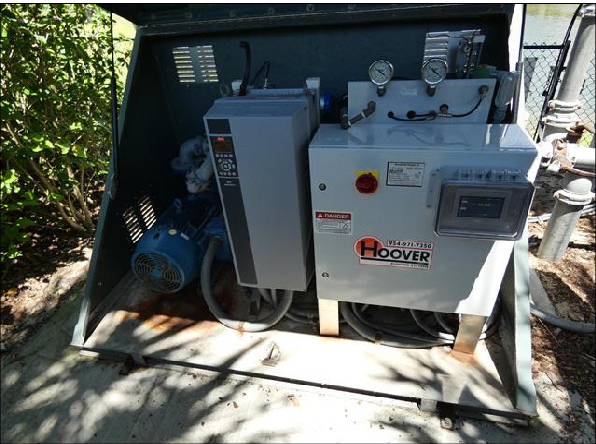
Pump Station 3 Carlsbad Dr
