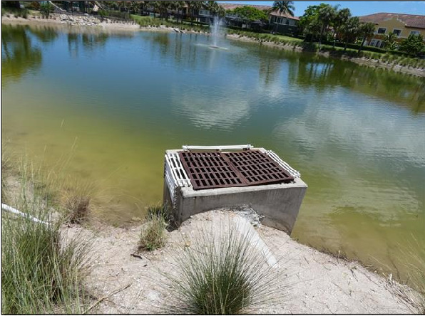
Stormwater Drainage Control Structure
