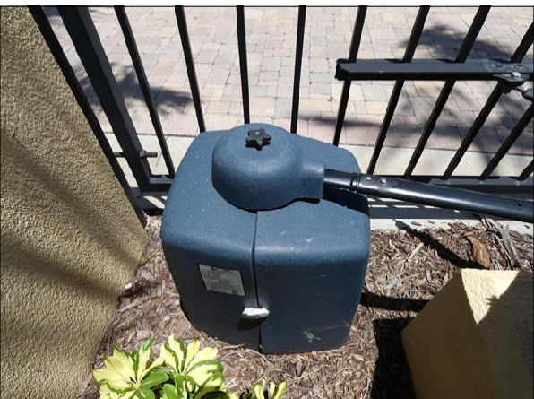
Palisades Dr Gate Operators
