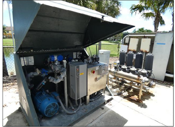
Pump Station 2 Near Playground
